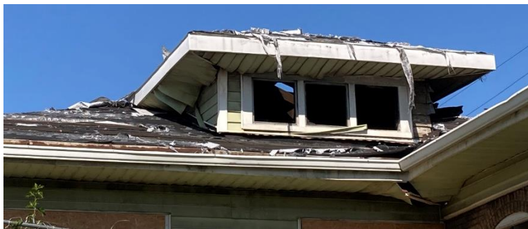
Front/south dormer showing hole in roof
