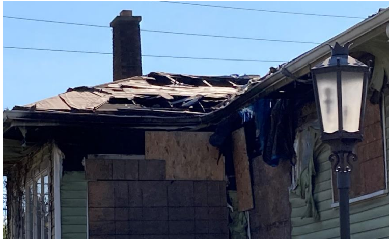
Holes in east side of roof
