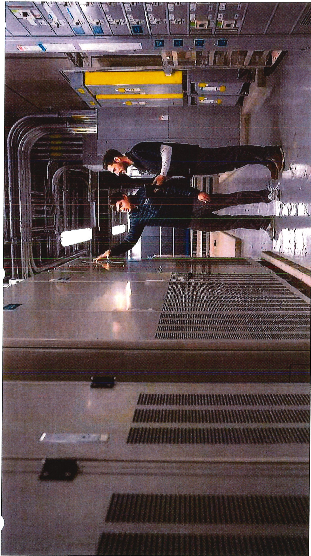
A photo provided by Sabey Data Centers shows the interior of one of the company's data centers. The Seattle-based company wants to build a data center complex near the intersection of Camby Road and Kentucky Avenue in Decatur Township. Credit: Provided photo/Sabey Data Centers
