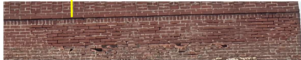
235: Damaged & missing bricks on upper level, below parapet/cornice; possible replacements
