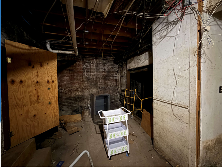
A: Abandoned freight elevator, non-functional
