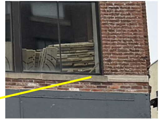
235: Dissimilar bricks on 1 st & 2 nd /3 rd floor indicating likely replacement; dissimilar pieces of stone on trim between 1 st & 2 nd indicating likely replacement
