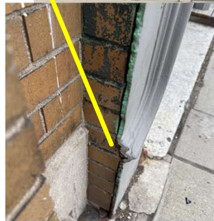
Cast metal at edge at 225 was roughly chopped off. May have been when 225 was rebuilt or when scored concrete façade was added
