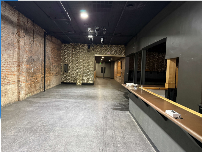
G: Front of former Tiki Bob's from entrance. Wall on right is the brick demising wall between 229 & 231. Columns support remaining portion of wall and carry weight of brick walls above, limiting sight lines and flow. Original brick demising walls were significantly altered by previous tenants, and no significant historic element remains.
