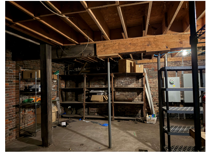
C: Storage area. Note additional support beams and sistered floor joists. Main beam was cut and jack installed under replacement. Floor is significantly higher than adjacent areas
