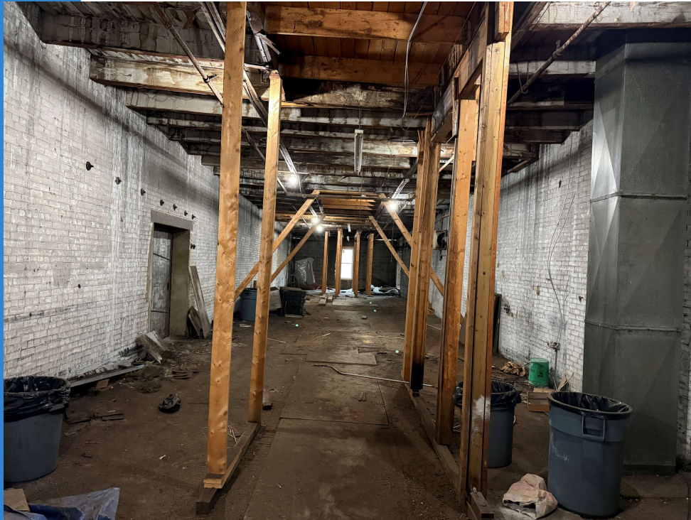
Z: Supports were added to support damaged roof. This area is above the section which was braced on 2 nd floor, indicating multiple levels of damage and neglect. Ceiling joists have been replaced but continue to sag.
