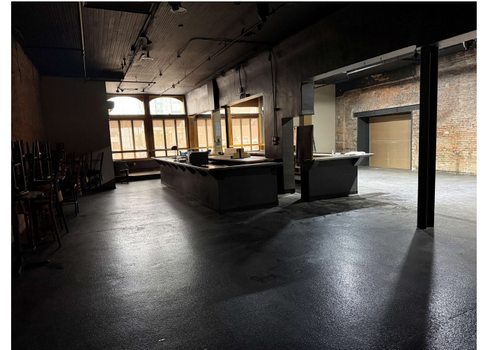
I: View toward Meridian Street. Dis-similar treatment on each side of the Meridian storefront.
