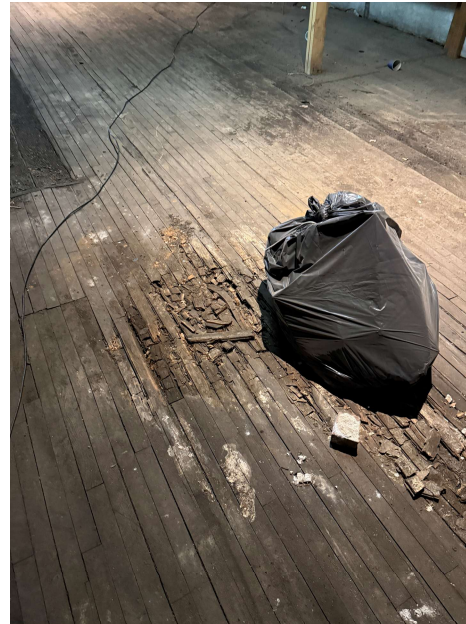
AA: Flooring has rotted and is crumbling in this area.
