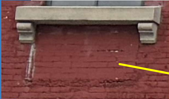
Brick replacement under window; likely dissimilar material; unmatched pattern
