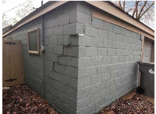
Structural Crack North
