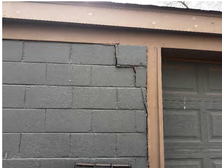
Structural Crack West
