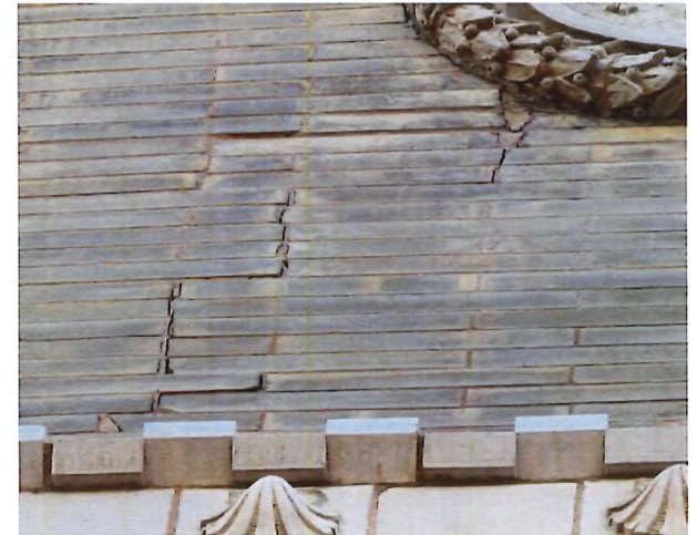
The face brick appear to be Roman in size ( 1 \frac{5}{8} " H x 3 \frac{5}{8} " D x 11 \frac{5}{8} " L). Cracking and displacement is present above the 2nd floor windows.
