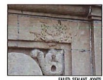
FAILED SEALANT JOINTS
