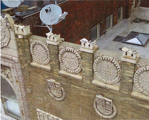
Monolithic construction of terra cotta, face brick and back-up brick to create the 15 N. Penn facade.
