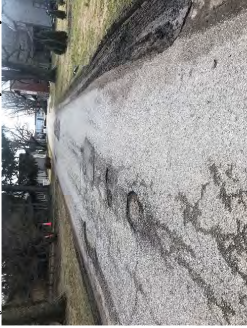
Image 4. Dobson Street just south of 73 rd & Dobson with yard destroyed by commercial traffic.
