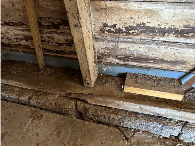
South wall crumbling foundation and remains of former support. Termite damage and rot present.
