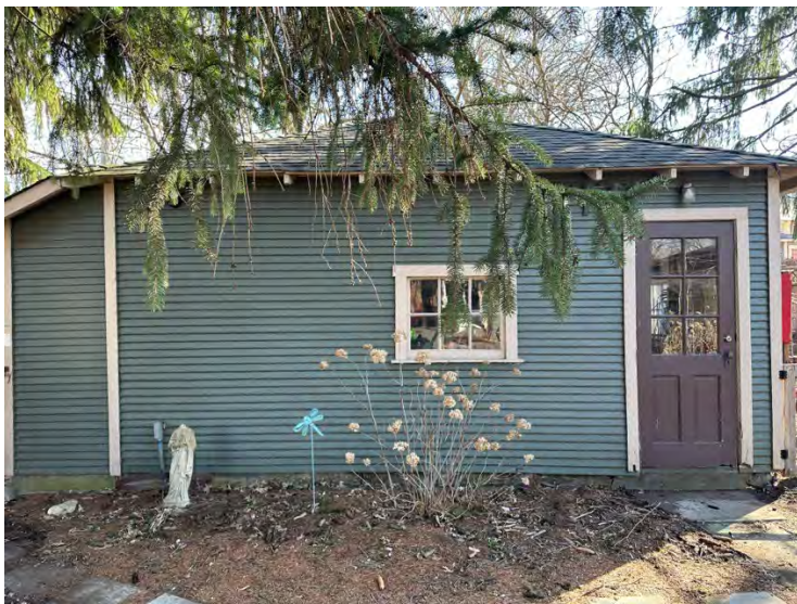
Overall view of North Wall/vehicle entrance. Uneven dirt floor and sagging structure.
