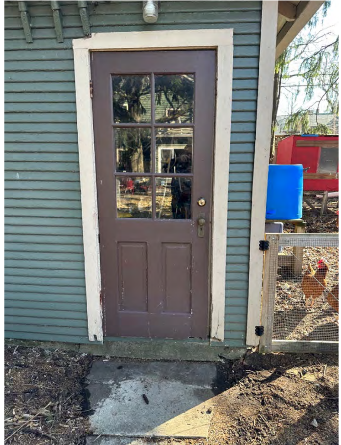
West Exterior: crumbling foundation and rotting trim.
