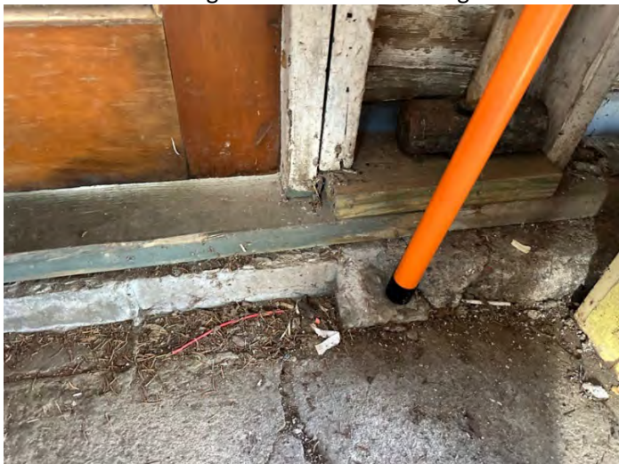
West wall crumbling foundation roof damage.
