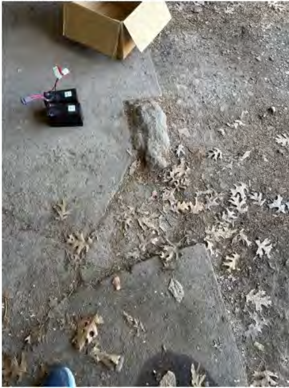
Slab doesn't extend to added construction:
