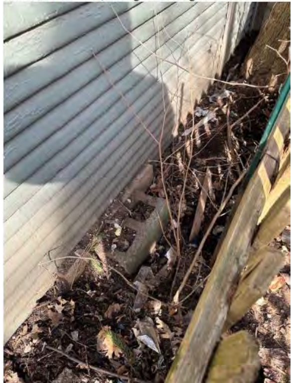
Outside of East wall, dirt against siding and holes in wall.
