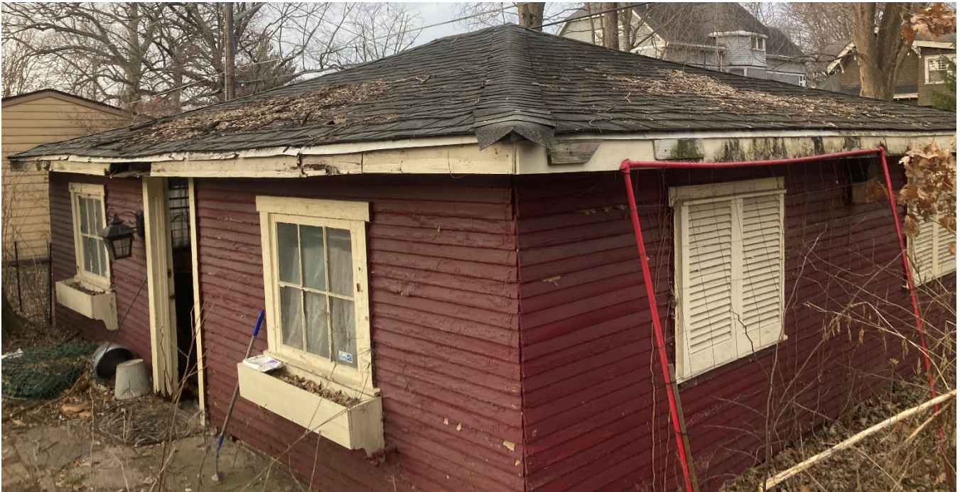
North and east façades. Walls are bowing and roof is falling.
