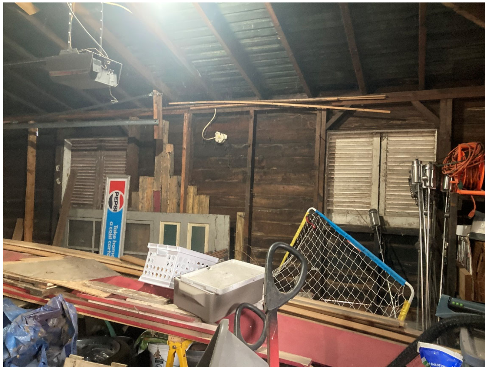
Missing windows on north elevation
