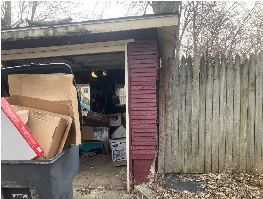
Notice bowing wall and foundation separation.
