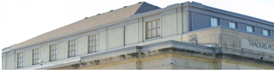
Northwest corner showing where shingles and exposed stucco material meet
