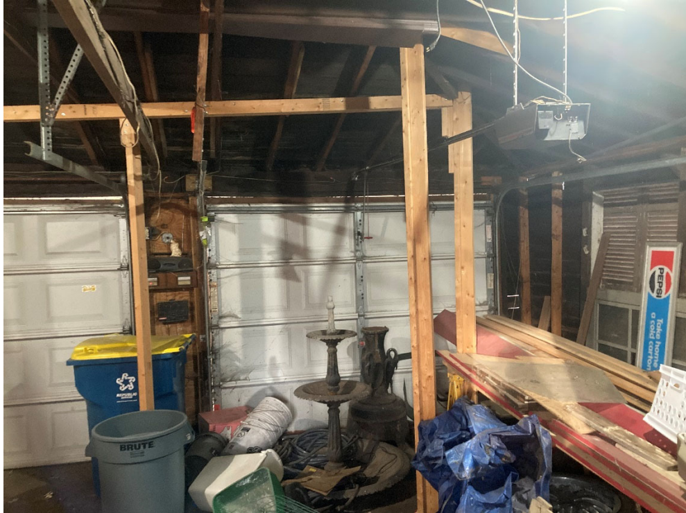
Makeshift 2x4 supports holding up western roof slope
