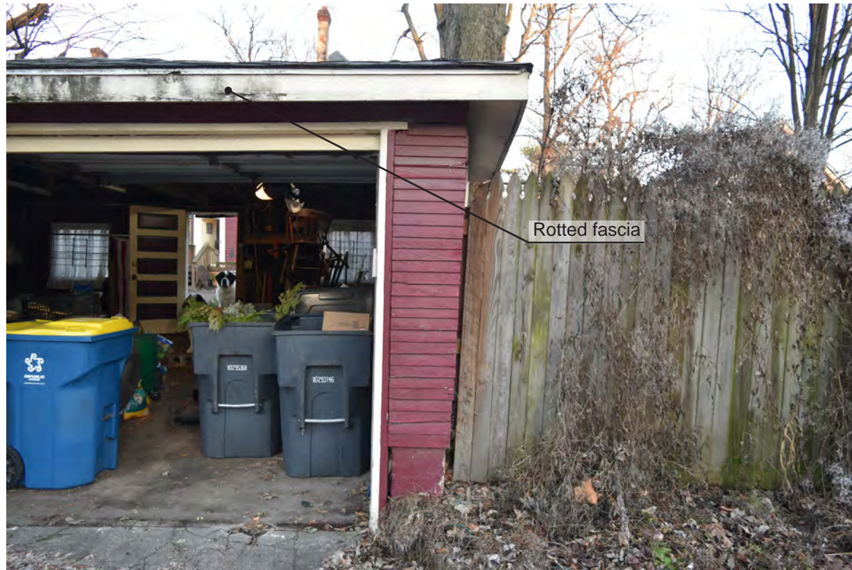
1 West facade of garage // wall out of plumb 5 See Image 1/6
