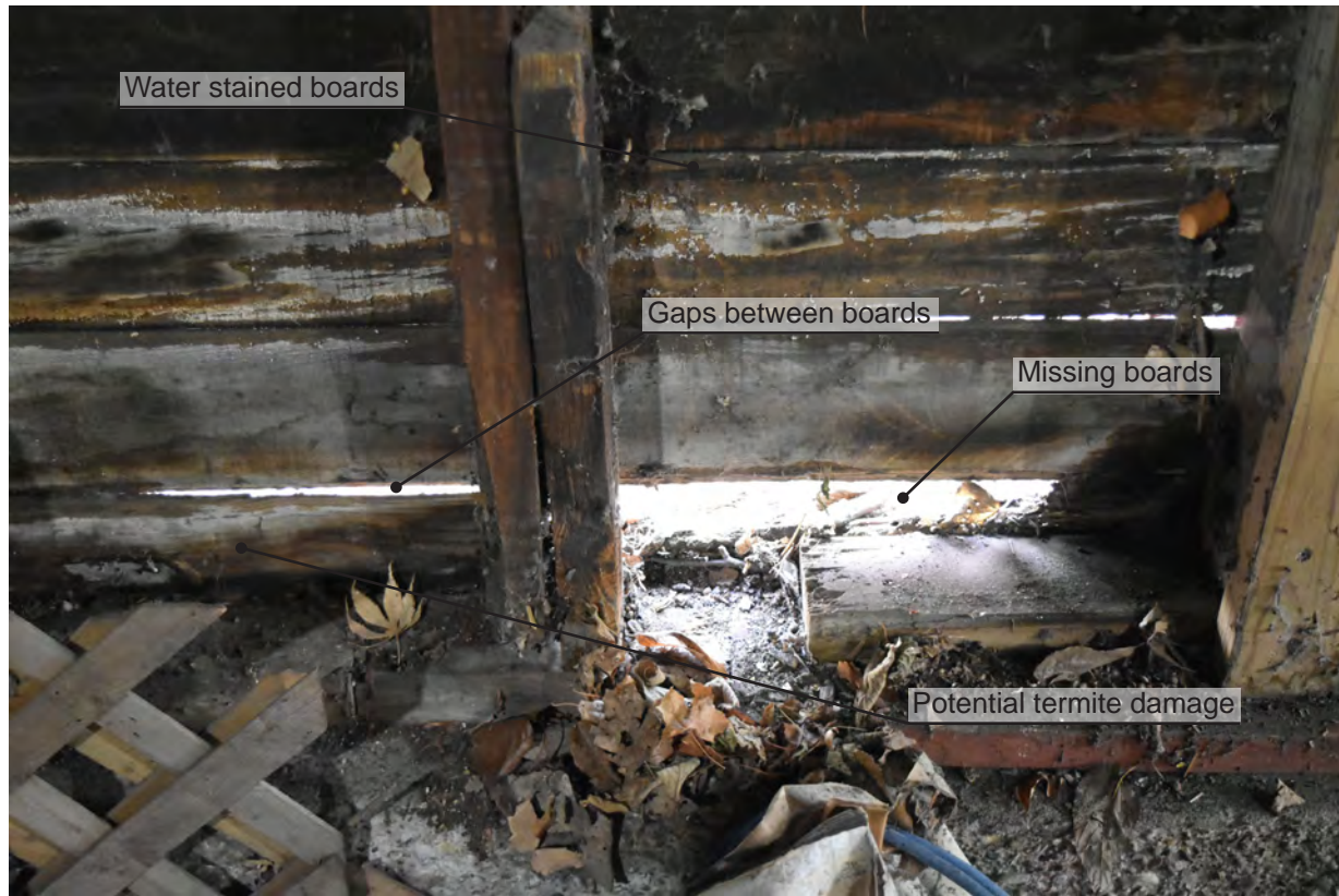
1 7 Garage interior // exterior siding deterioration
