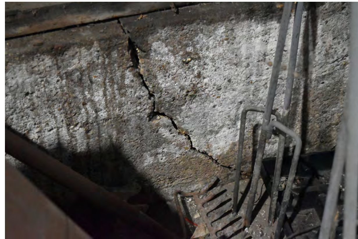
2 Garage interior // cracks in the foundation 5
