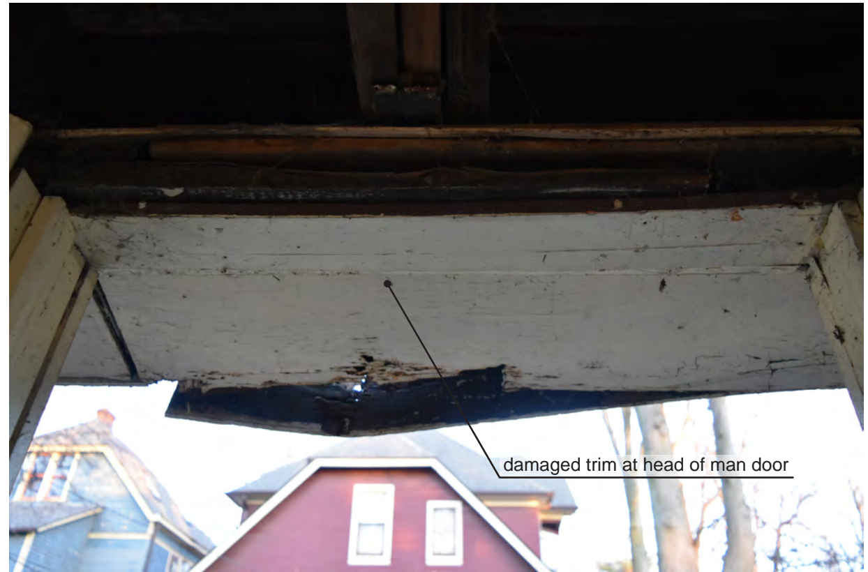
2 18 Deteriorating soffit and door jamb of garage door
