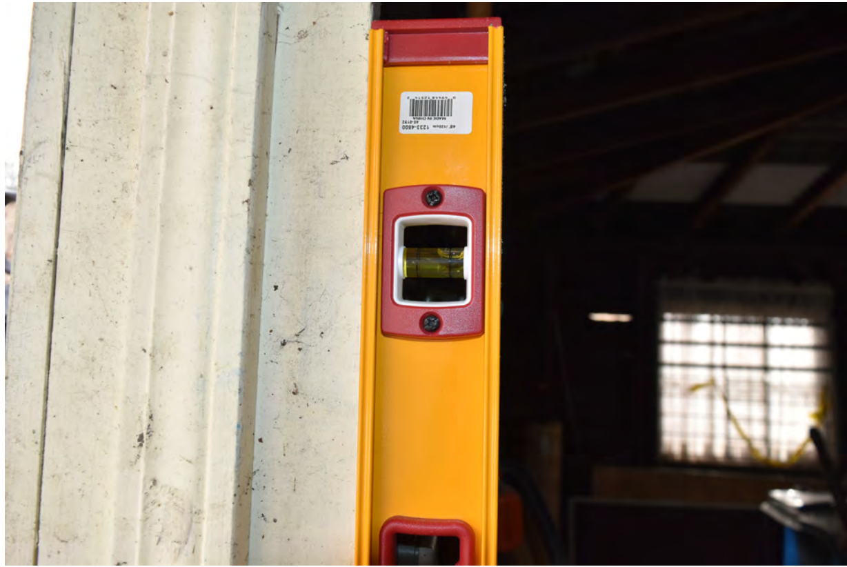
1 6 Garage door frame out of plumb
