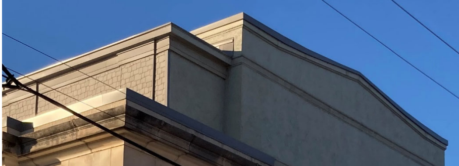
Southeast corner showing where shingles and exposed stucco meet
