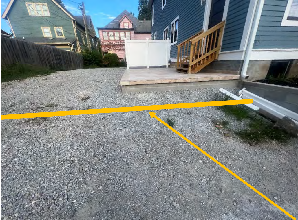
Looking east at rear yard space prior to sod installation. Extension of wall here.
