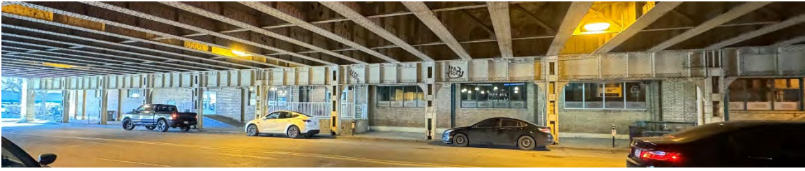
Illinois Street Bridge (left north elevation, right south elevation also showing train shed)
