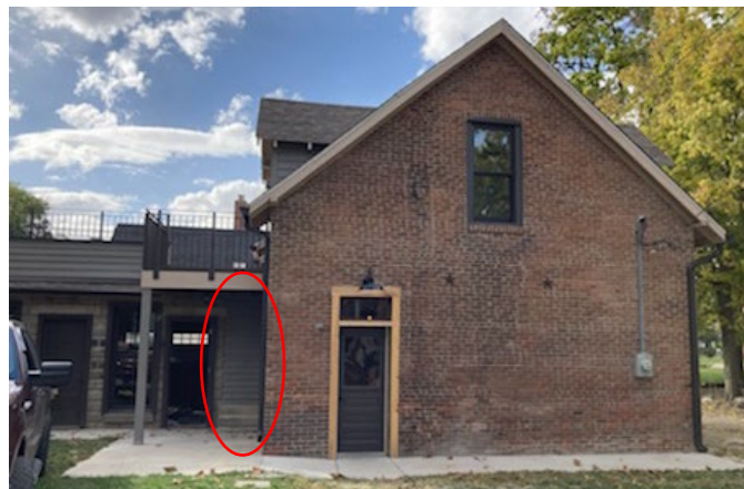
View of east side of brick carriage house and concrete block garage – showing location of infill (circled)
