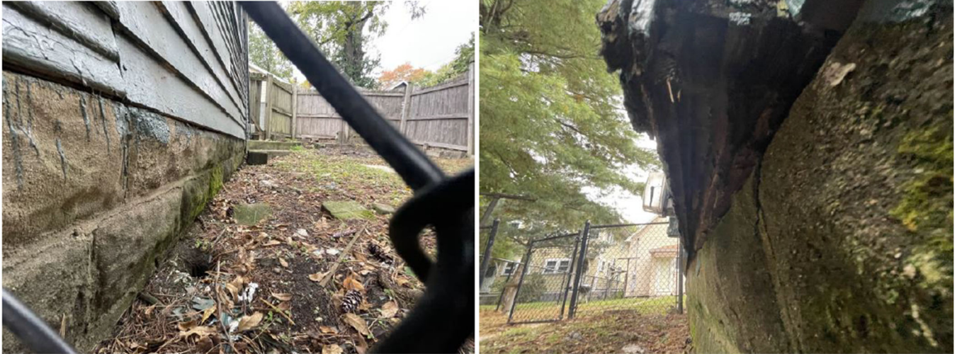
From engineer's report: examples of out of plumb foundation and exterior wall
