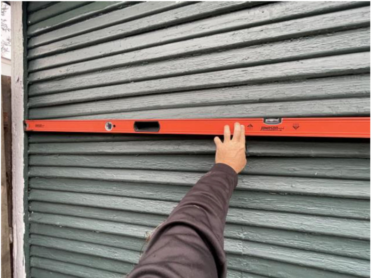
From engineer's report: example of severely out of plumb wall
