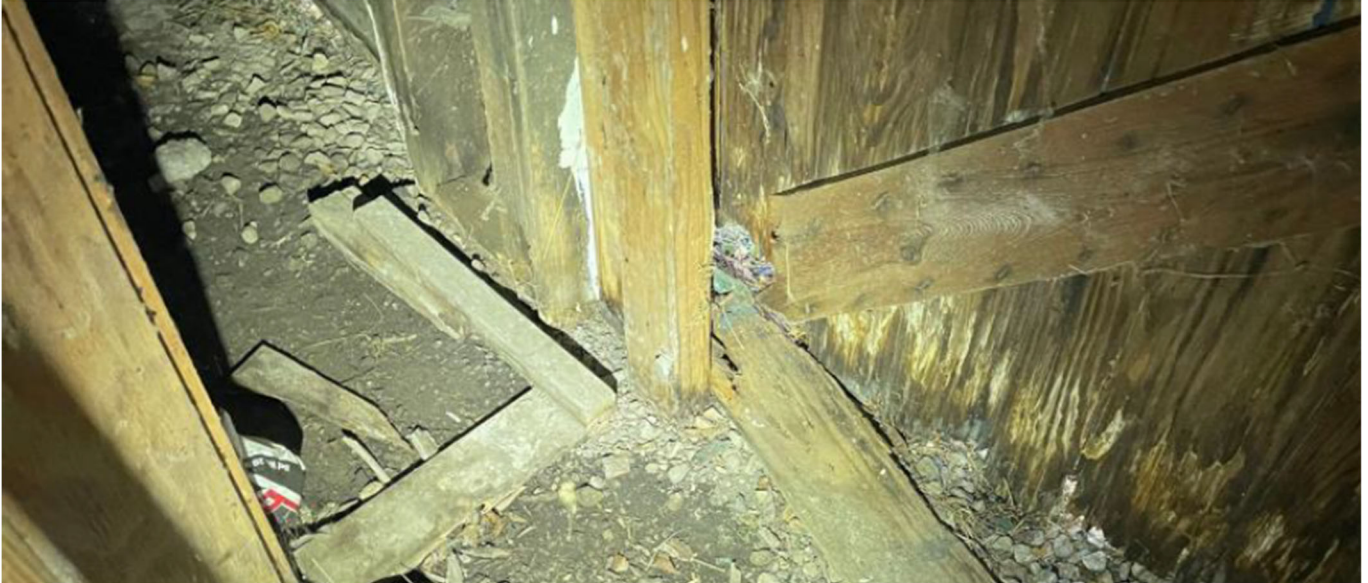
From engineer's report: example of deteriorating wood framing sitting directly on the ground
