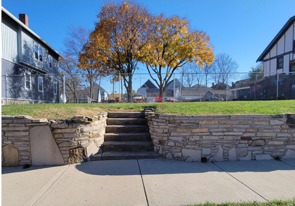
2135 N Alabama – historic retaining wall. (runs across the front of 3 lots total)
