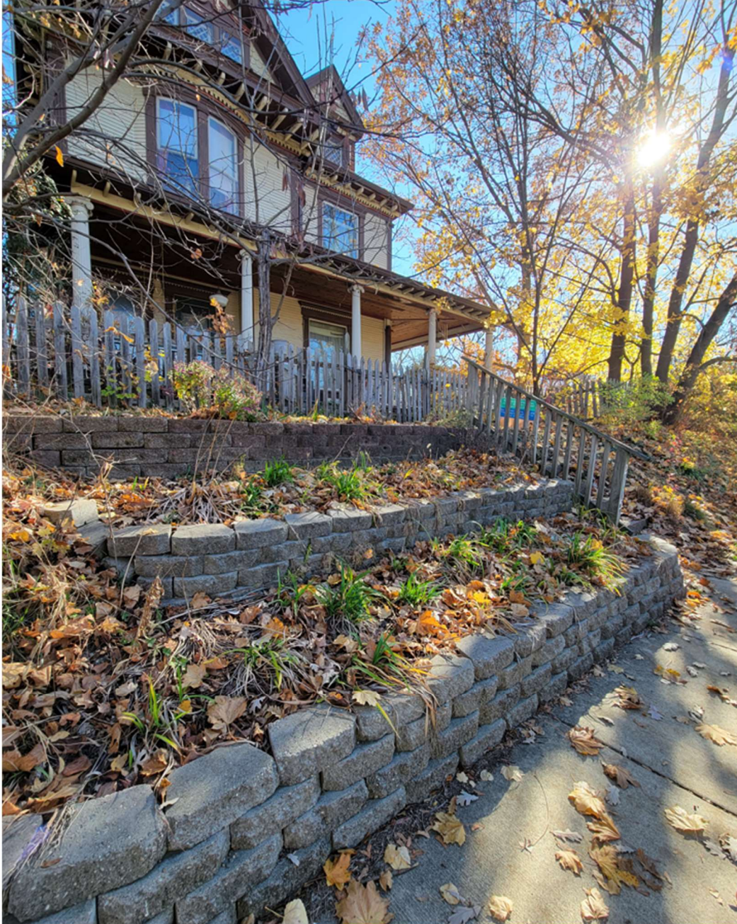
2115 N Alabama (directly north of the 21 st & Alabama street intersection). Retaining wall with (3) tiers & front fence.
