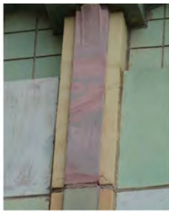
PREVIOUSLY REPAIRED CRACK
