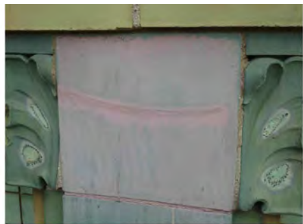
PREVIOUSLY REPAIRED CRACK
